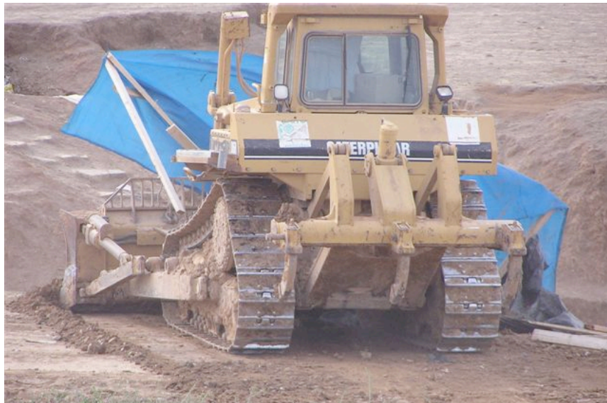
Picture 1: Bulldozer of the Jewish National Fund demolishing a shack in Al Arakib on February 9, 2011.
