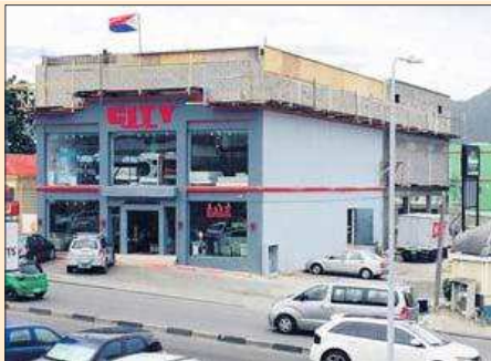
The expansion of the City Furniture building on Bush Road has reached its highest point.
