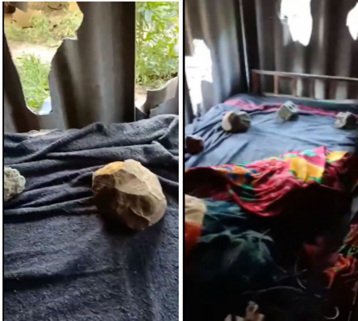
The rocks thrown through the walls of Mrs. TTĐ's house
