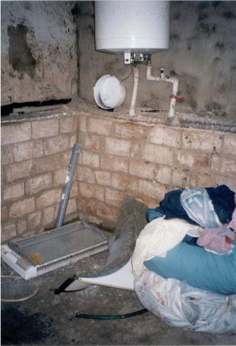
Bathroom facilities with a boiler in the house in Stará Červená Voda in the Jeseník District, Czech Republic, 13 May 2007, to which two families were deported by the Vsetín municipality after being expelled from municipal housing without procedure in November 2006.
