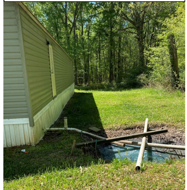
Image: A pool of raw sewage from straight pipes collects behind one resident's home in Lowndes.
