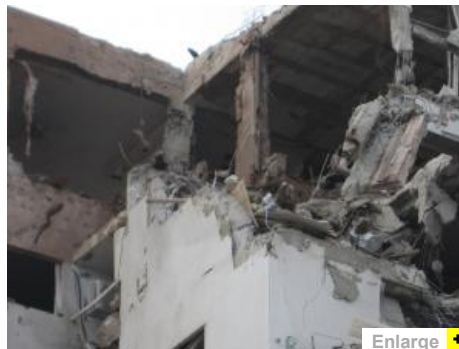
Several apartment buildings in Rishon LeZion, outside Tel Aviv, were damaged by rockets fired from Gaza.
